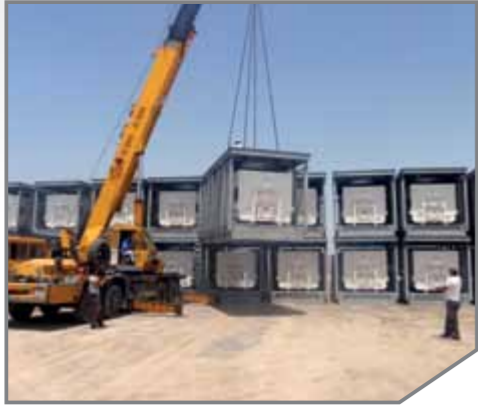
platform and compactor storage
